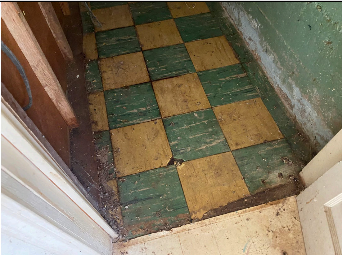
View of multi-layered ACM Floor Tile and Mastic – Lower Level Common Room, Rooms 131, 132, 133, 134, Lower Level Storage Room #2
